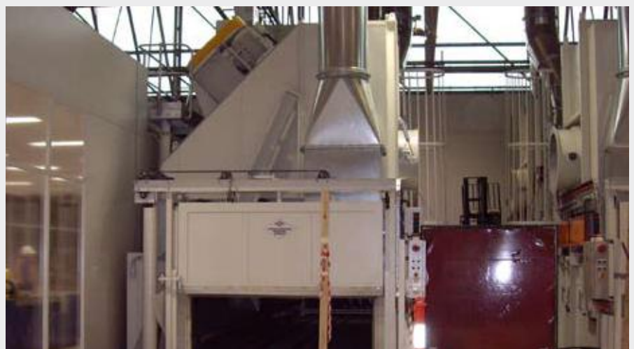
First oven commissioned for curing 787 skins.
